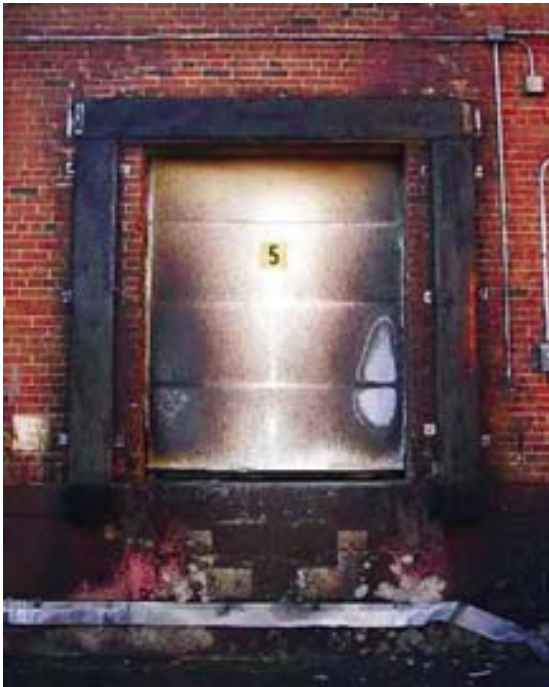
Dock-seal fire damage caused by truck-trailer marker lights.
